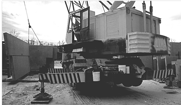
When a crane begins to tip, the back end becomes light and rises into the air. This places stress on the crane's components and can cause structural damage, including boom collapse. In addition, adequate blocking should be placed under all outrigger pads and the crane's swing radius should be barricaded.
