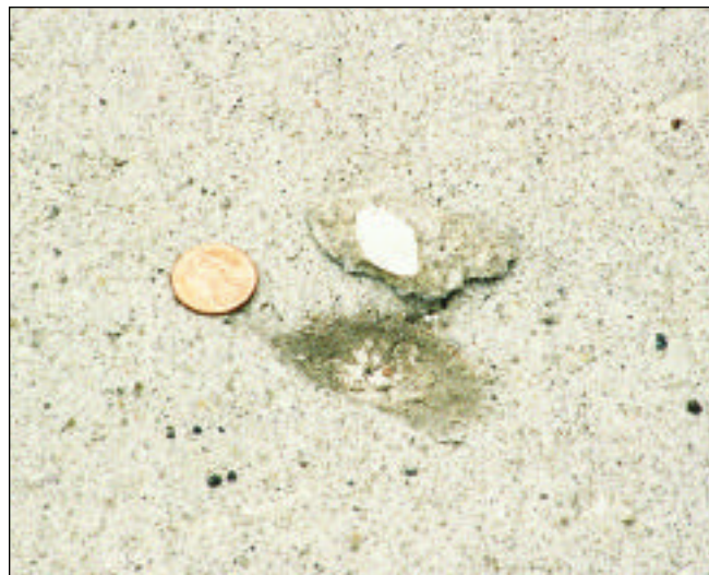
Popouts are ¼ inch to several inches in diameter, and usually a portion of aggregate remains at the bottom of the hole.
